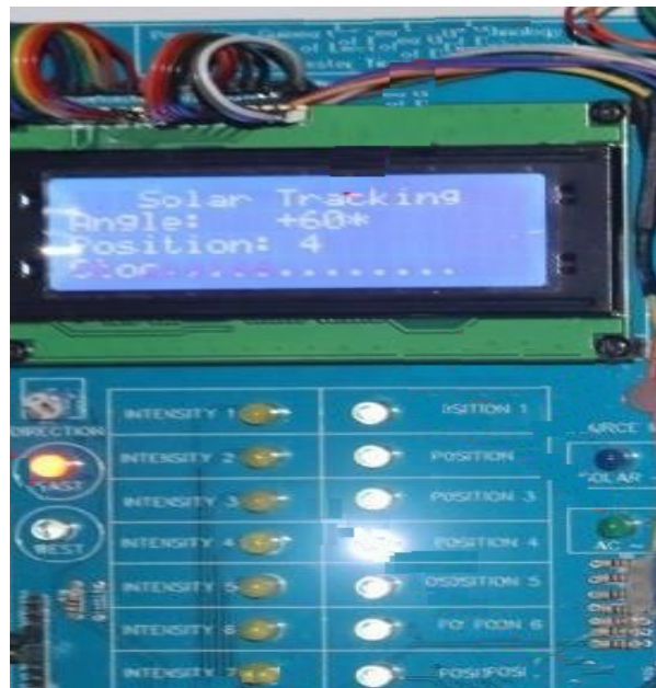
Fig. 11. Display panel of the single-axis solar tracker.
